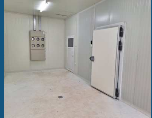
SEPARATE ELECTRICITY METERS
