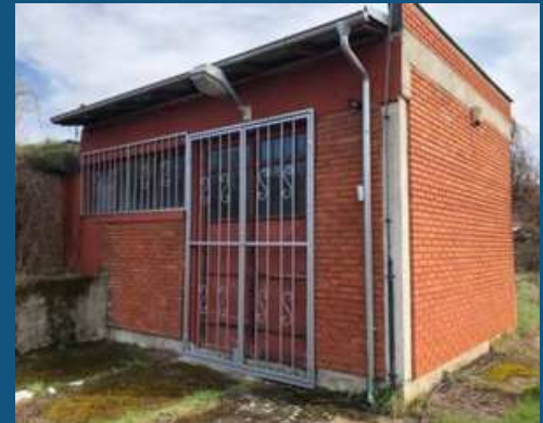
ONSITE WATER PUMP
